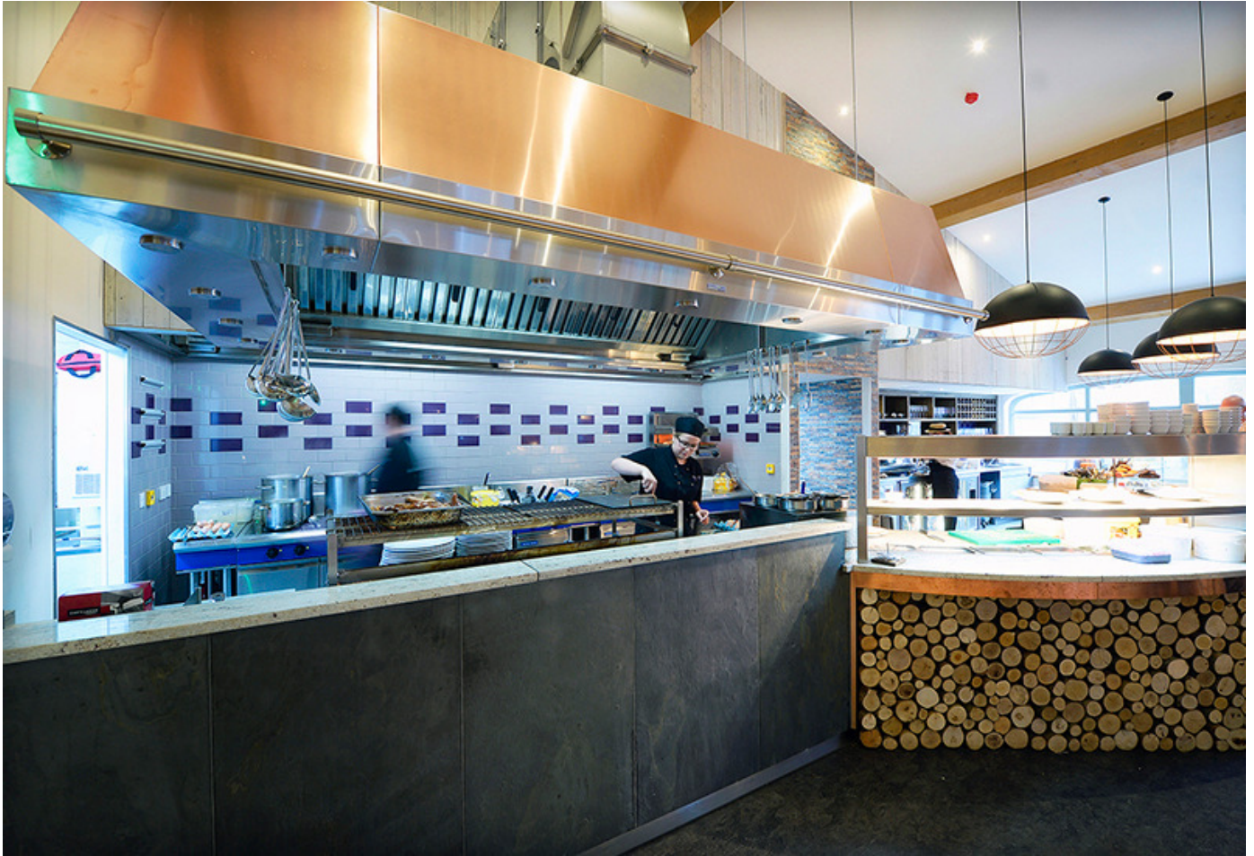
Moo and Beast feature a theatre kitchen designed and installed by CDG.
